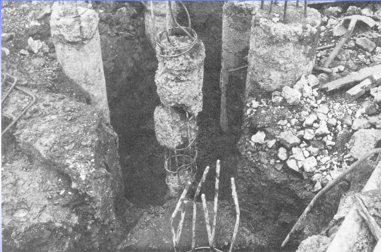
Effective shaft of bored pile due to washing out of cement of unset concrete
